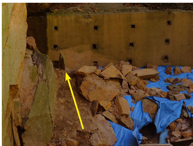
Figure 33: Disturbance at the base of the lower retaining wall noted by John Clarke, President of the Société Jersiaise and Dr Peter Chowne during the site visit on 18 April 2013
