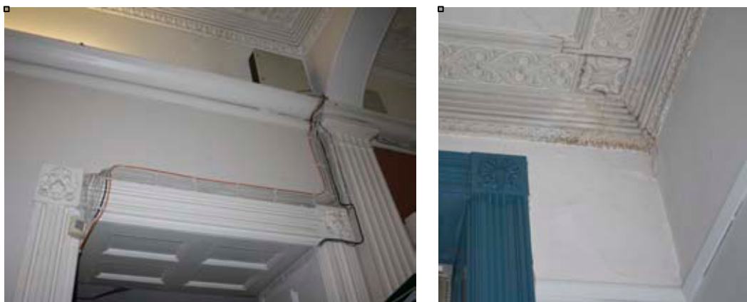
Figure 2.1 a. Cabling around doorframes in ground floor hall is both physically and visually damaging to the historic fabric b Isolated occurrences of damp should be carefully monitored.
