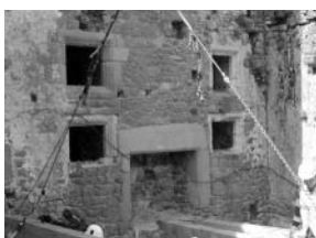
As the English Oak floor beams are airlifted in by helicopter, the workmen carefully put them into place in the Great Chamber.
