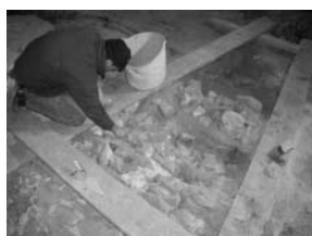
Repair work being carried out on the floor of the Medieval Great Hall.
