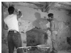
The restoration of plasterwork in the lower level of Prynne's Tower by French stonemasons.
